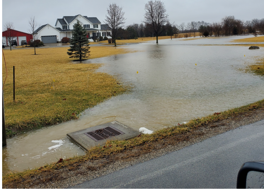
Figure 2: Evidence of surface flooding at 8604 Carter Road, facing north. This photograph was taken on February 22, 2022, after a 1.2 inch rain event.
